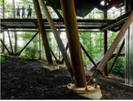
Weathering steel recalls the cultural heritage of the site and visually integrates with vertical forest elements. - Photo Credit: Photography by Joe Fletcher
